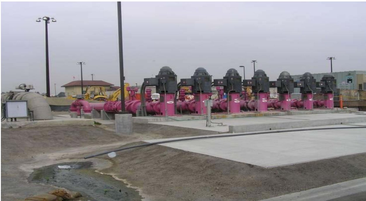
RP-1 South Zone Pump Stations Source: Inland Empire Utilities Agency
